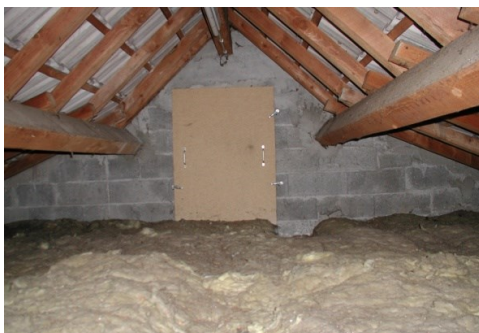
Glass-fibre insulant, outmoded and useless when damp!
